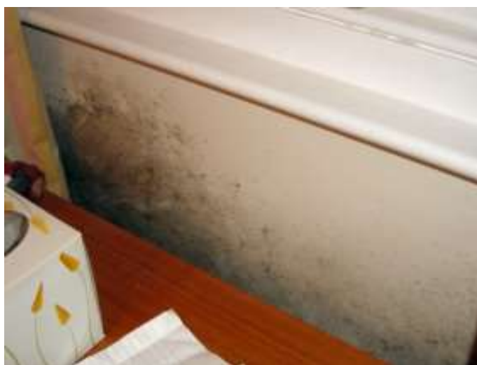
Condensation leading to black mould growth behind a dressing table.
