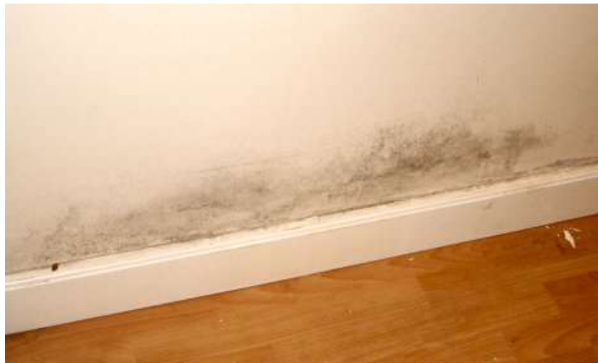
Condensation and mould at skirting boards level, commonly mistaken for rising damp
