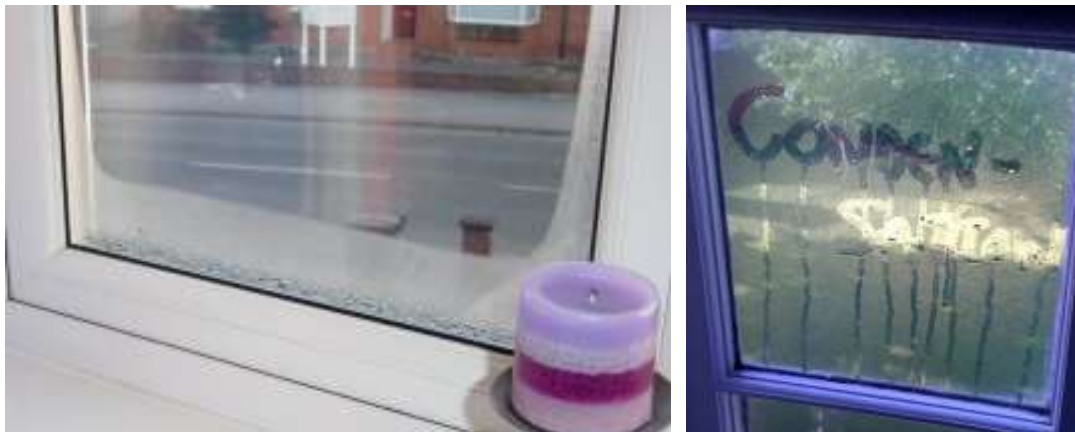
The above show condensation occurring on windows, both double glazed and single glazed
